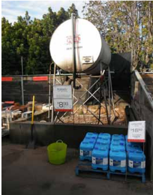
Photo 9– Fuel tank and chlorine pallet
